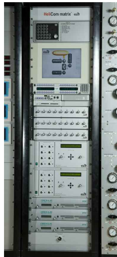
HeliCom™ Matrix Communications System
